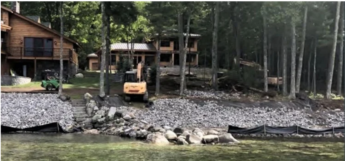
An excavator works on shore at 18 Fernwood Road on Sebago Lake in this photo taken October 2021. Town of Raymond photo
